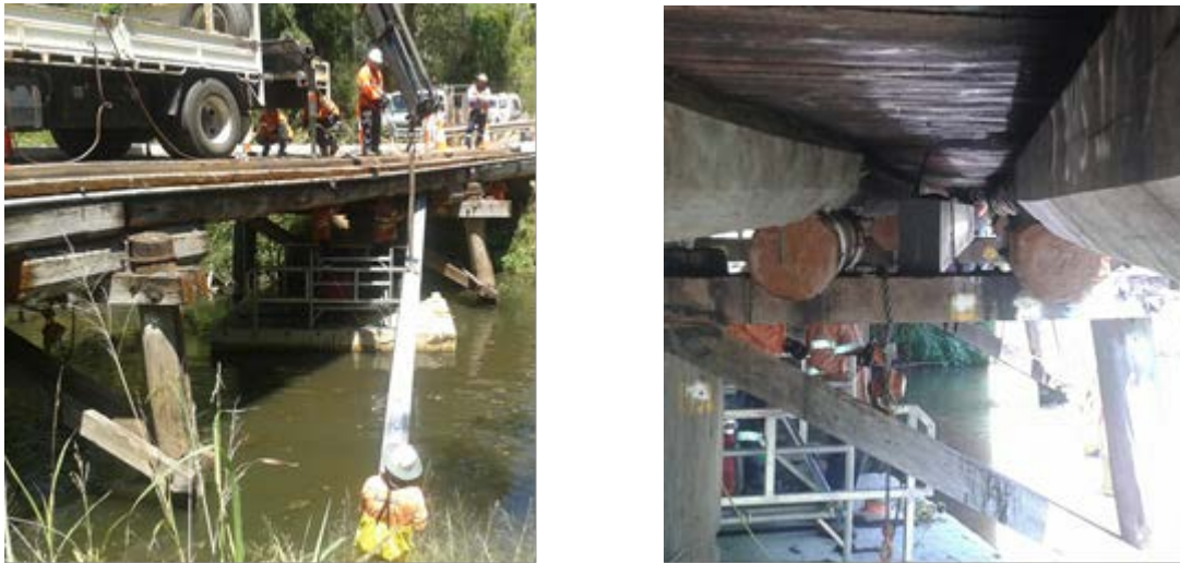
Figure 10.5a - Loc's FRPC girder lifted under bridge (left) and positioned beside faulty timber girder (right)
