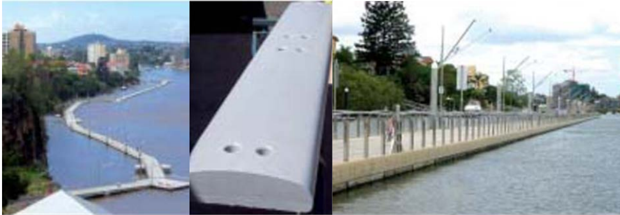
Figure 5b - FCDD's fibre composite waler beam used in the BCC River Walk Project
