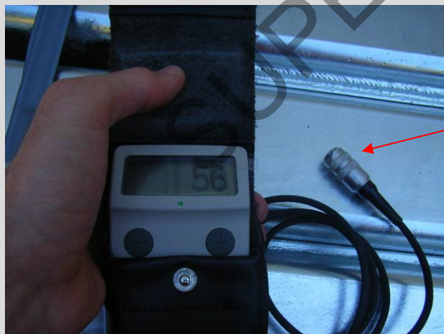
Figure 11.3.1(a) – View of the low coating thickness
