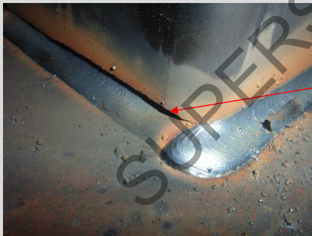
Figure 8.5.6(e) – View of the undercut in the post
