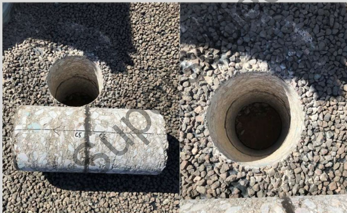
Figure 8.9.9.4.3 – Core showing the C170 spray seal interlayer bonding the plant-mixed foamed bitumen stabilised layers together
