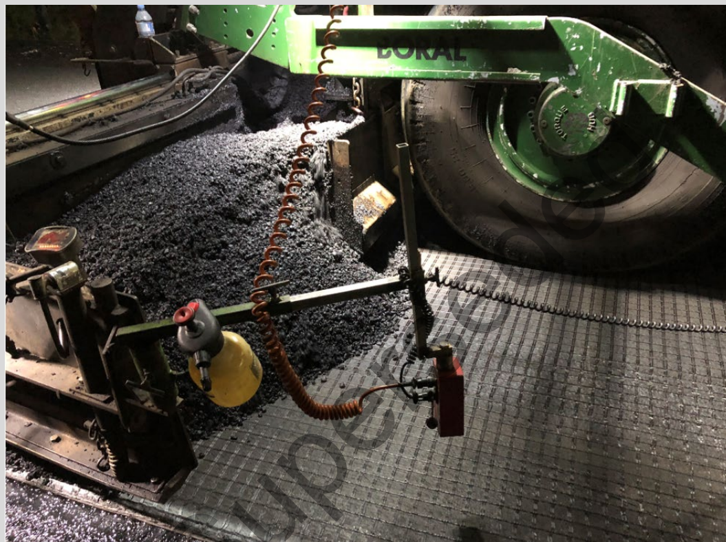
Figure 9.4.1 – Example of asphalt being paved on asphalt geosynthetic with no bow-waves, wrinkles or folds
