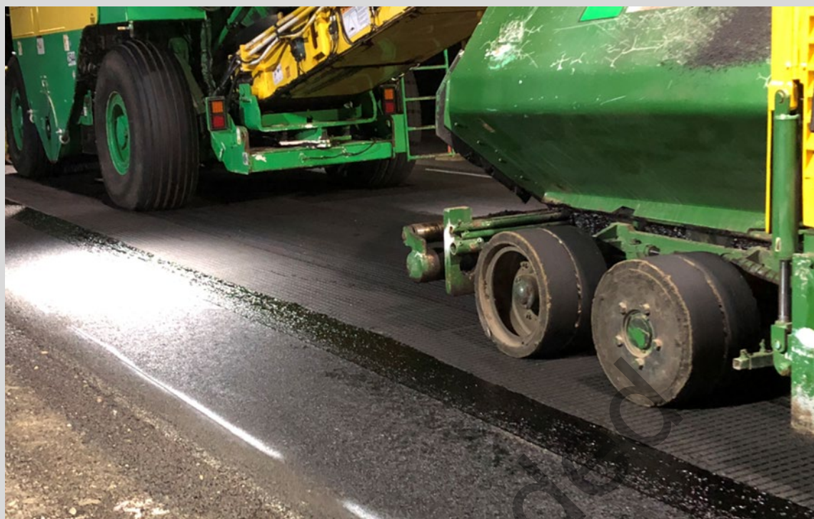
Figure 9.4.2(c) – Example of minimum bitumen pick-up on truck tyres or paving equipment
