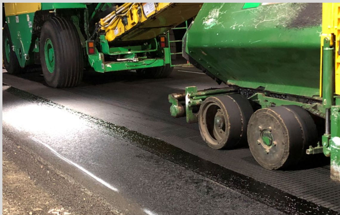
Figure 9.6.3(b) – Minimum bitumen pick-up or wrinkling of the asphalt geosynthetic under the construction plant
