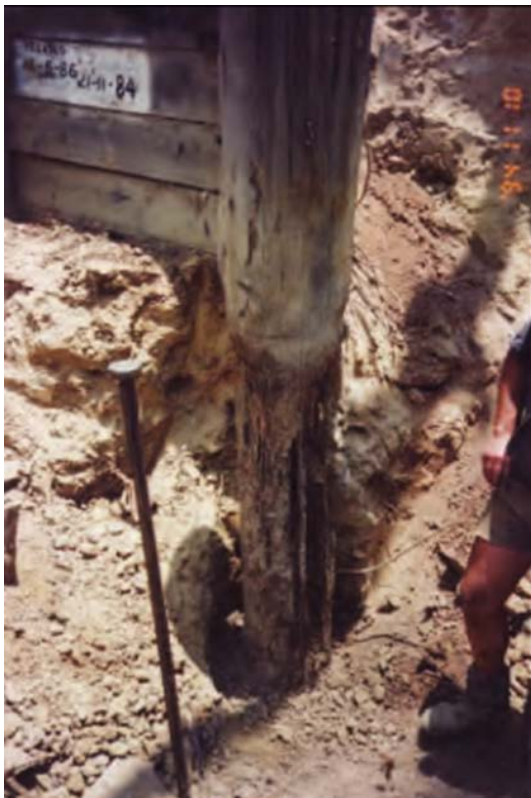
Figure 3.3.5a – Decay of pile below ground level
