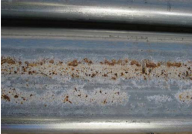
Figure 2.3.2a – White deposit on zinc metal spray
