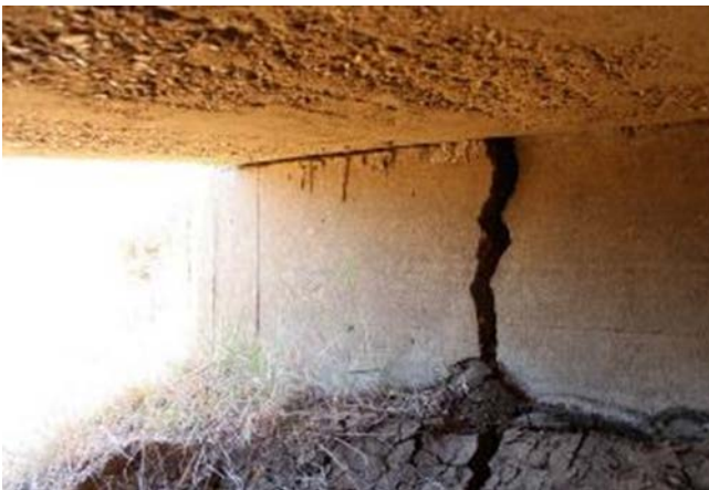
Figure 2.2.3.2c – Crack/separation in abutment wall due to differential settlement
