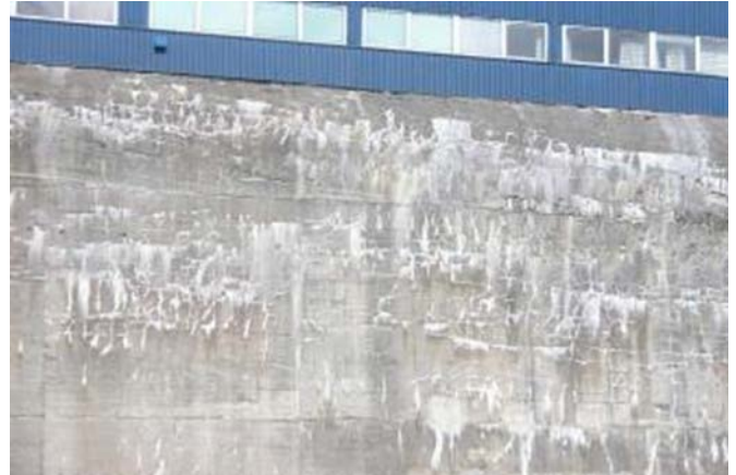
Figure 2.2.6d – Discharge through cracks in concrete surface
