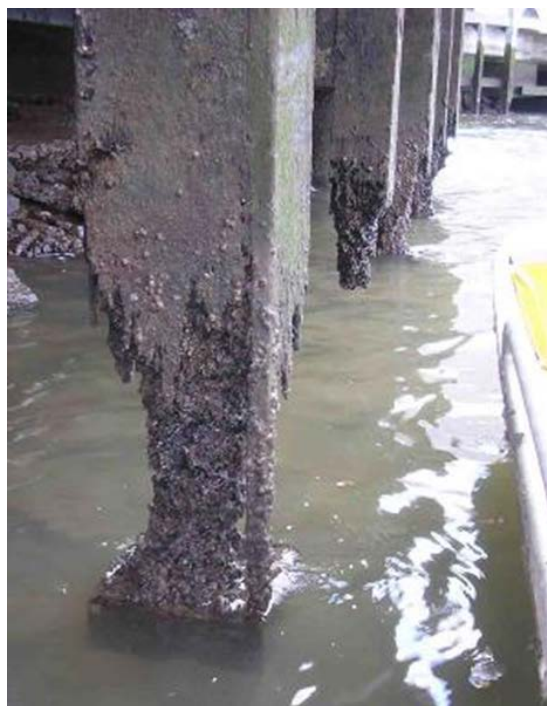
Figure 2.4.3b – Timber piles subject to Sphaemora attack
