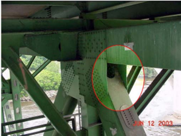
Figure 2.3.3a – Buckling of gusset plate
