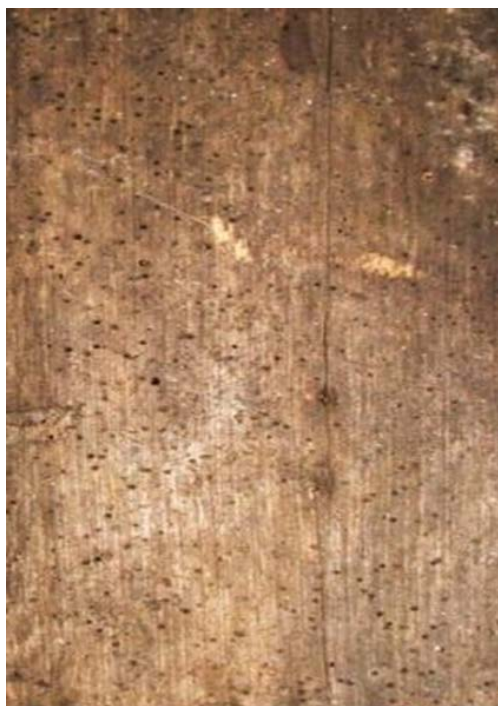
Figure 2.4.3a – External damage to timber pile from shipworm
