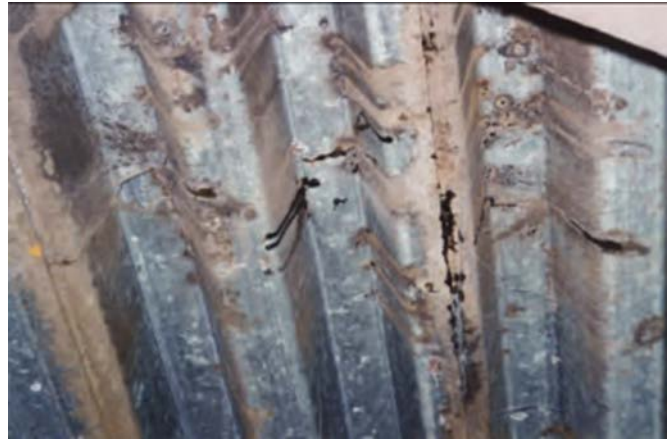
Figure 3.3.3.4b – Cracking and perforation of steel trough decking
