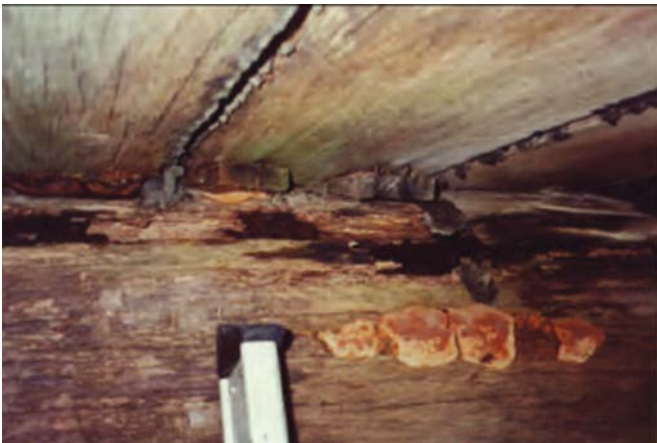
Figure 2.4.1a – Fungal fruiting body and decay of girder
