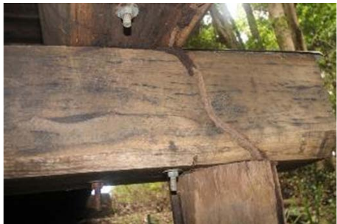
Figure 2.4.2b – Termite gallery on pier headstock
