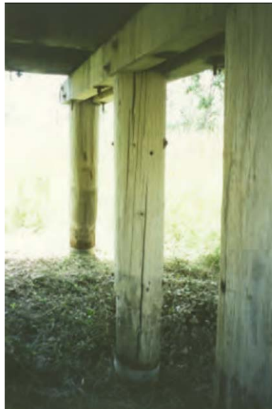
Figure 3.3.5b – Splitting of pile beneath headstock
