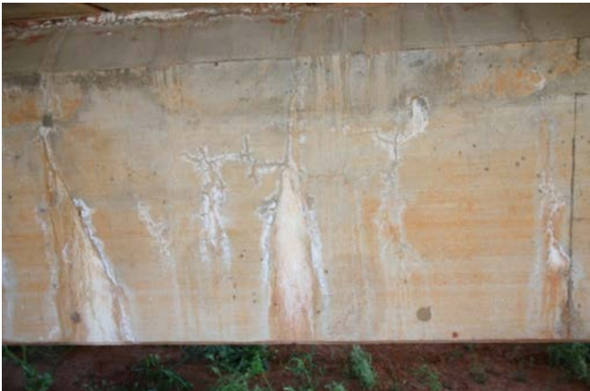
Figure 2.2.6c – Efflorescence evident on concrete headstock
