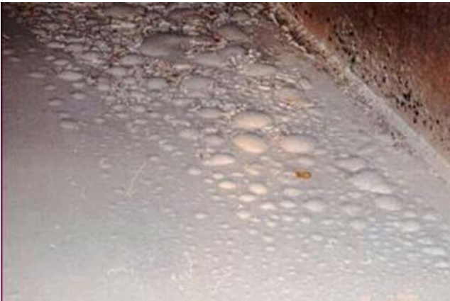
Figure 2.3.2c – Blistering of paint system
