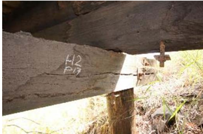
Figure 2.4.4.1b – Splitting in timber headstock
