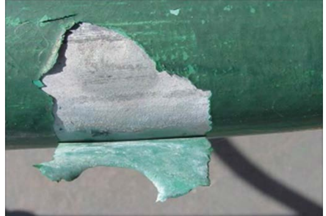
Figure 2.3.2b – Failure of paint system over galvanising
