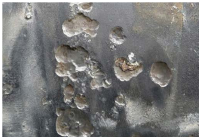
Figure 2.3.1d – Corrosion of steel by SRB
