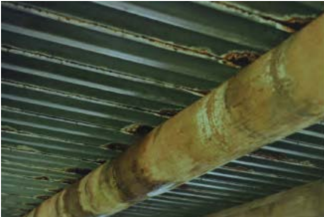
Figure 3.3.3.4a – Corrosion of joints between trough sections
