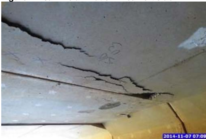
Figure 2.2.6a – Delamination in culvert slab
