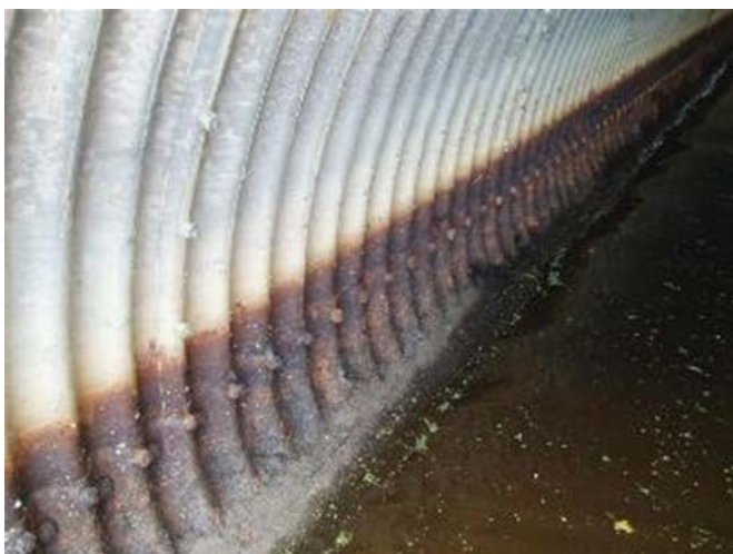
Figure 3.4.2.2a – Typical location of wall corrosion in BCM culvert
