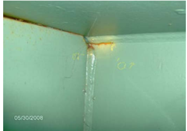
Figure 2.3.4b – Cracking in welds
