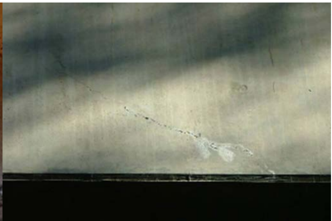
Figure 2.2.3.2d – Shear crack in girder adjacent to support
