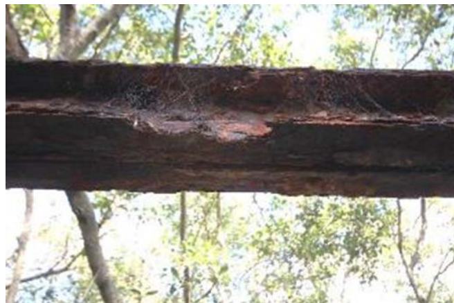
Figure 2.3.1b – Severe corrosion and loss of section
