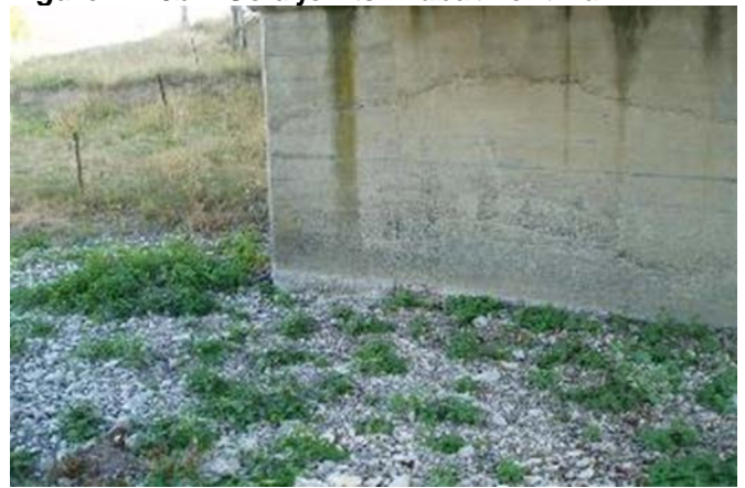
Figure 2.2.6b – Cold joints in abutment wall
