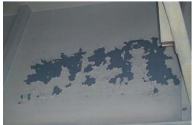
Figure 2.3.2d – Flaking of paint system
