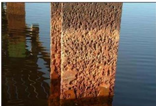
Figure 2.3.1c – Pitting of steel
