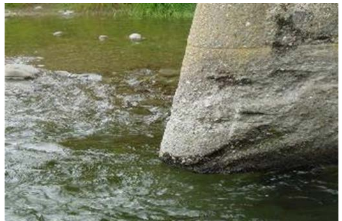
Figure 2.2.6f – Abrasion of concrete
