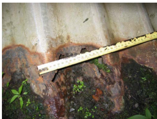
Figure 3.4.2.2d – Perforation of BCM culvert wall
