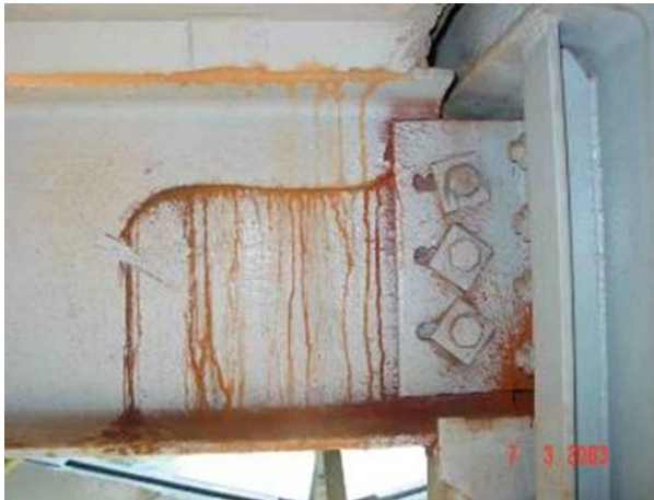
Figure 2.3.4a – Fatigue cracking in web
