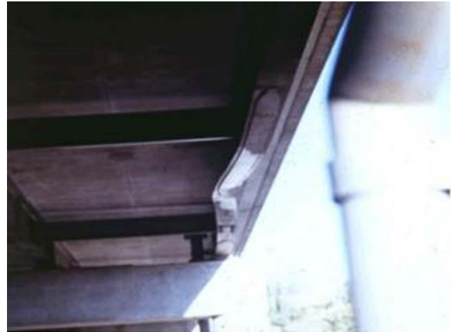
Figure 2.3.3b – Impact damage to steel beam
