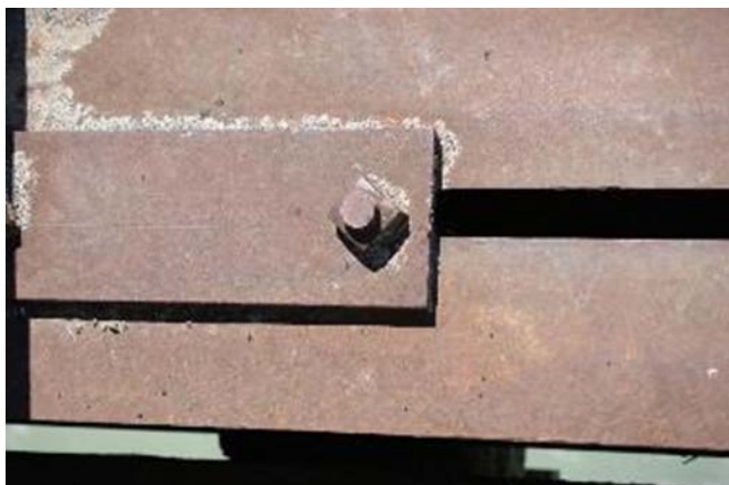
Figure 2.3.1a – Mild surface corrosion
