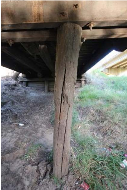
Figure 2.4.4.1a – Splitting in timber pile
