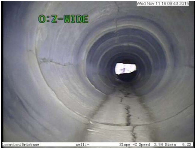
Figure 3.4.2.1a – Cracking of pipe walls
