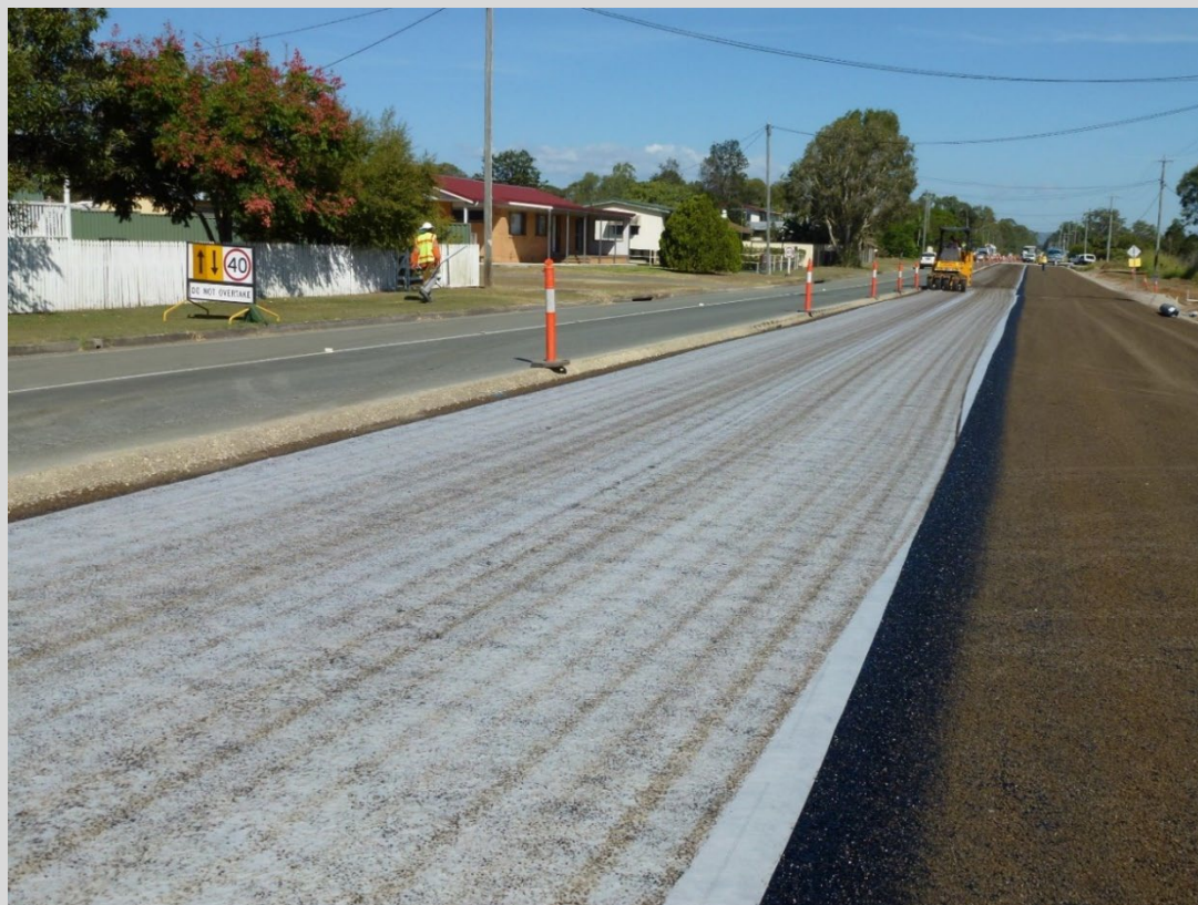
Figure 8.7.3(a) – Rolling geotextile using a multi-tyred roller to help impregnate the bitumen into the geotextile.
