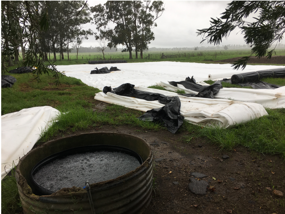
Figure 1 - 600R Geotextile being pre sewn into 36m x 20m panels (Nelsons Plains)
