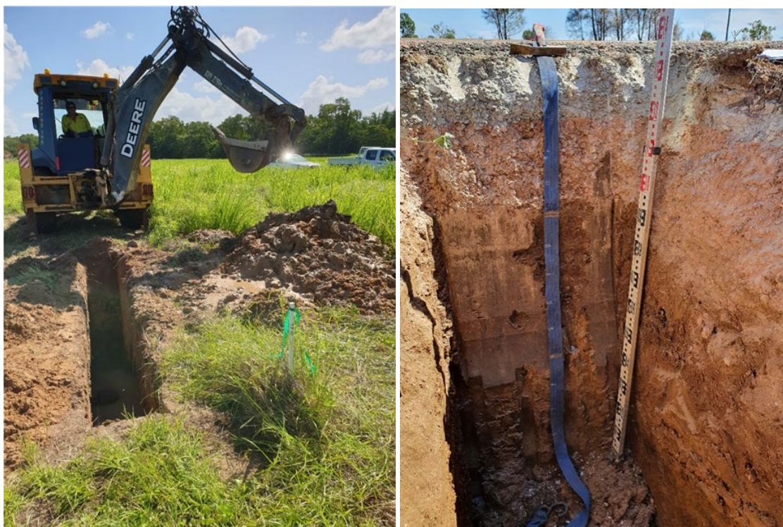
Figure 4.4.5(a) – Example of excavating test pit (left) and test pit profile (right)
