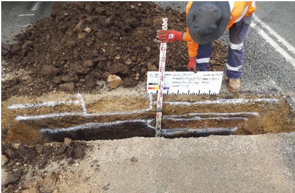
Figure 4.4.4(b) – Example of trenching showing the high level of pavement profile detail
