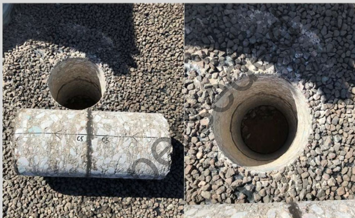
Figure 8.8.9.4.3 – Core showing the C170 spray seal interlayer bonding plant-mixed foamed bitumen stabilised layers together
