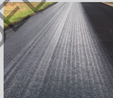
Unacceptable binder uniformity
