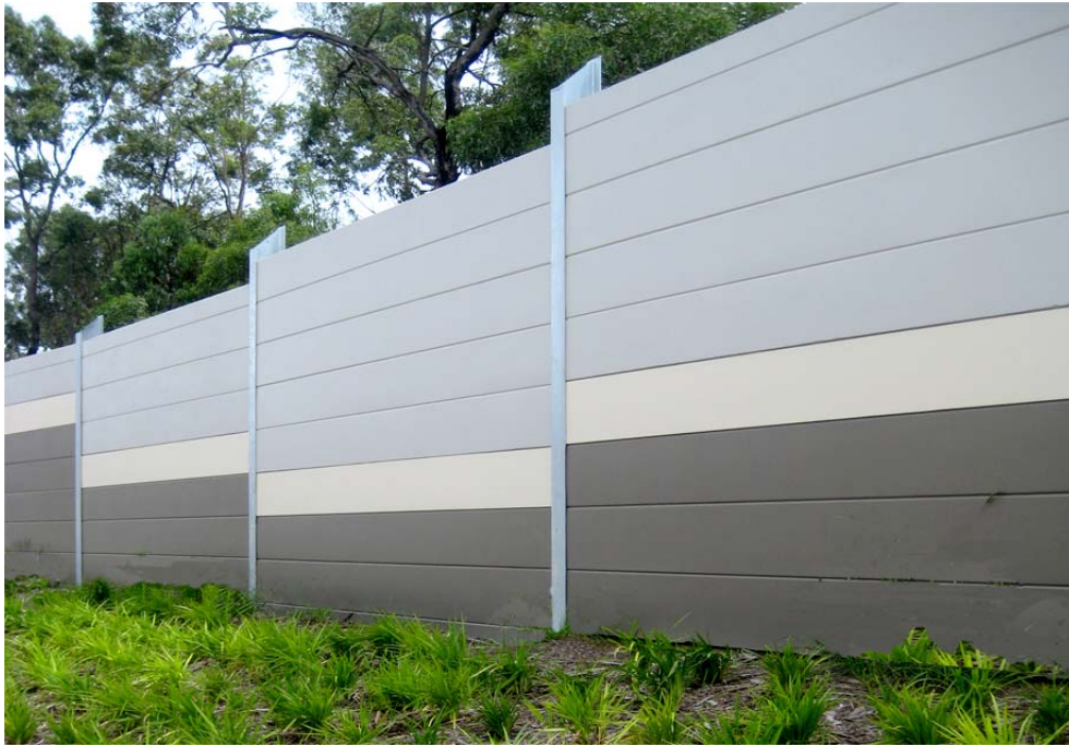
Figure C3-7: Colour and pattern in conjunction with material selection used in noise barriers design to create visual interest and express corridor themes
