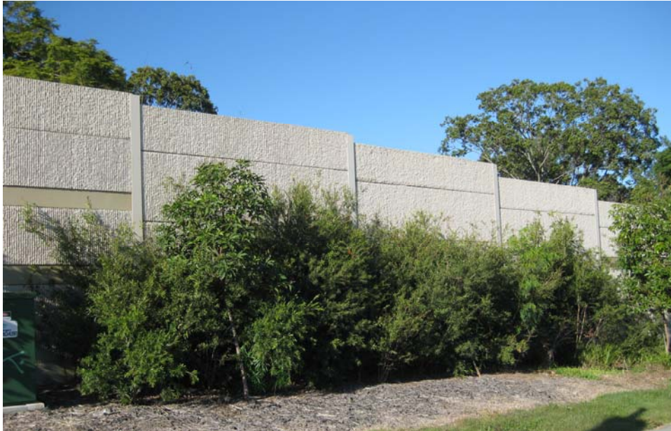
Figure C3-6: Buffer planting protecting noise barrier from vandalism and graffiti
