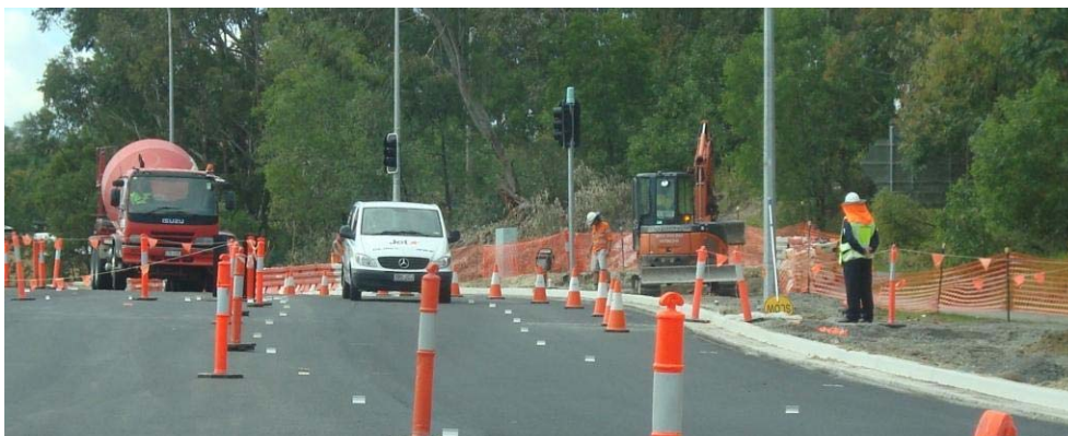
Figure D1-3: Effective traffic control in place to ensure safety of personnel maintaining road landscape
