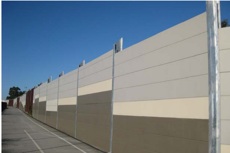
Figure A4-20: Universal design components, like noise barriers that fit together to achieve a road function
