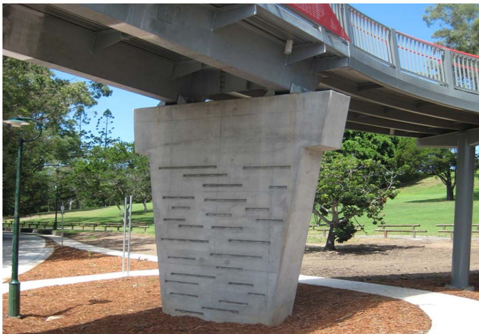
Figure C3-2: Tapered and textured piers create a visually recessive structure within the road landscape
