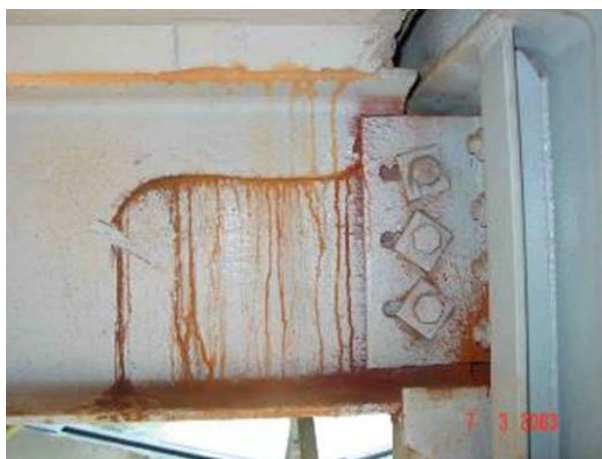
Figure 2.3.4a – Fatigue cracking in web
