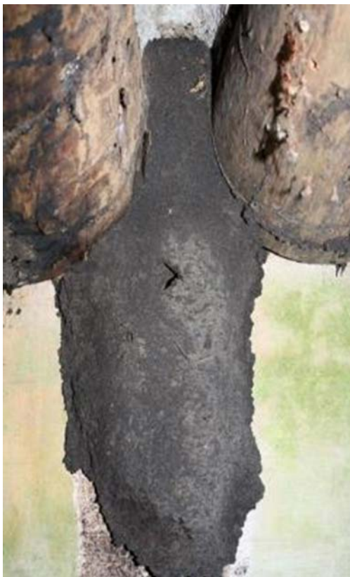
Figure 2.4.2a – Termite nest on bridge pile
