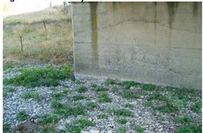
Figure 2.2.6b – Cold joints in abutment wall
