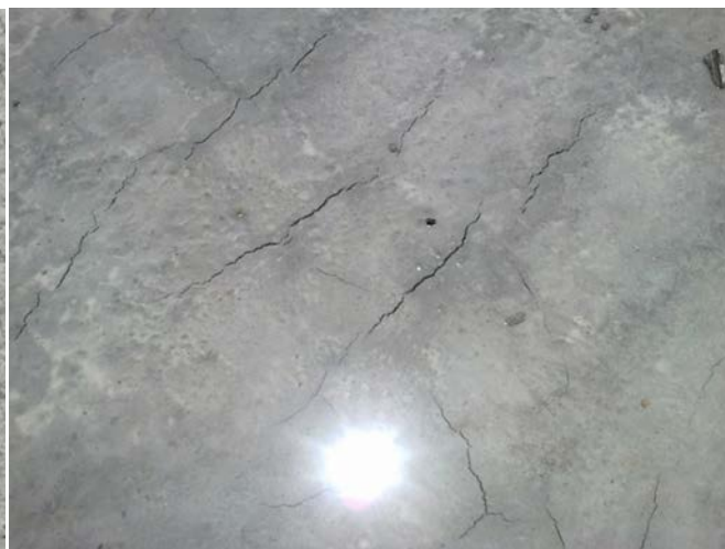
Figure 2.2.3.1c – Plastic settlement crack in slab
