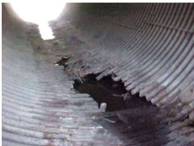
Figure 3.4.2.2c – Perforation of BCM culvert invert
