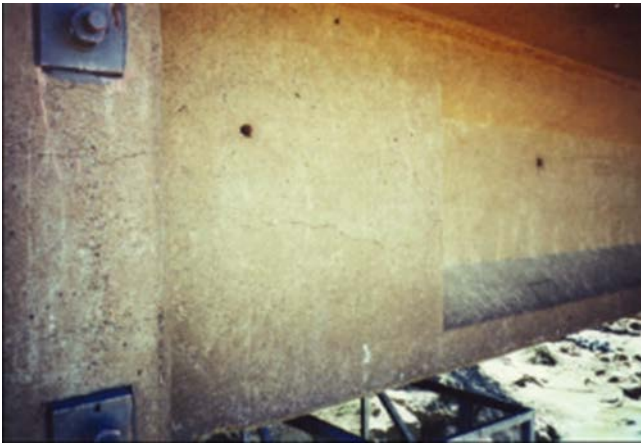
Figure 2.2.3.2a – Bursting cracks in under-reinforced anchorage zone of post-tensioned girder
