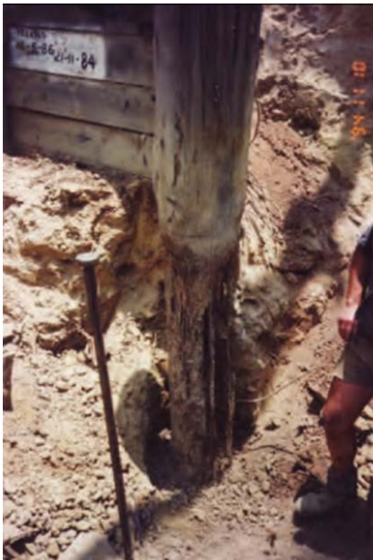
Figure 3.3.5a – Decay of pile below ground level
