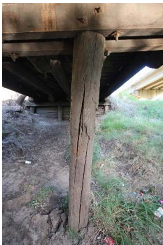
Figure 2.4.4.1a – Splitting in timber pile
