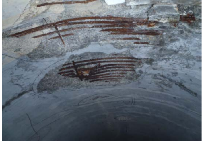
Figure 3.4.2.1b – Loss of cover/spalling concrete in pipe crown
