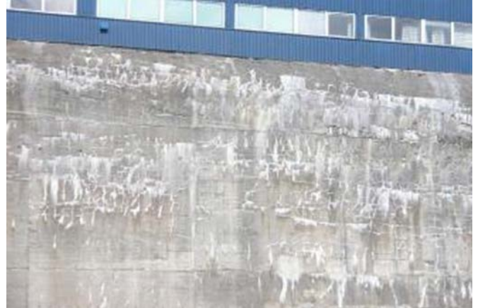
Figure 2.2.6d – Discharge through cracks in concrete surface
