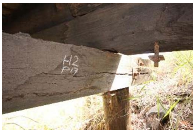
Figure 2.4.4.1b – Splitting in timber headstock
