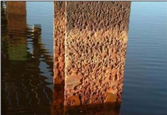
Figure 2.3.1c – Pitting of steel
