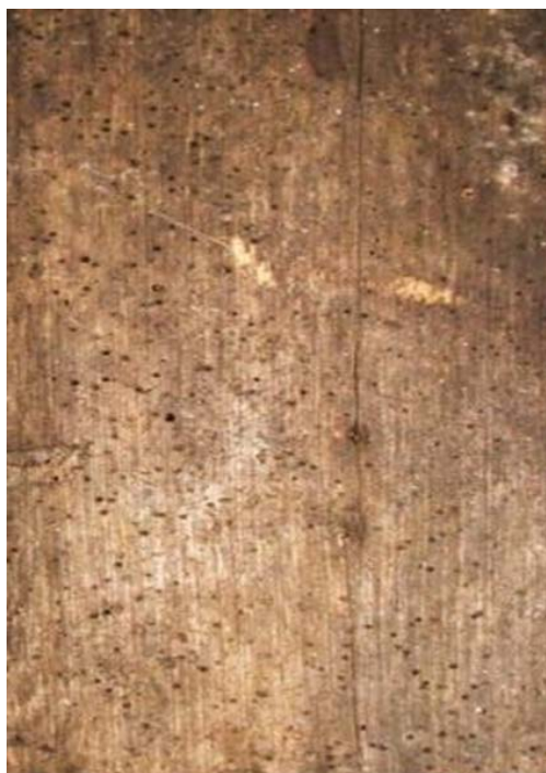
Figure 2.4.3a – External damage to timber pile from shipworm
