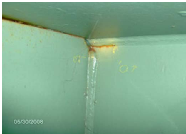
Figure 2.3.4b – Cracking in welds
