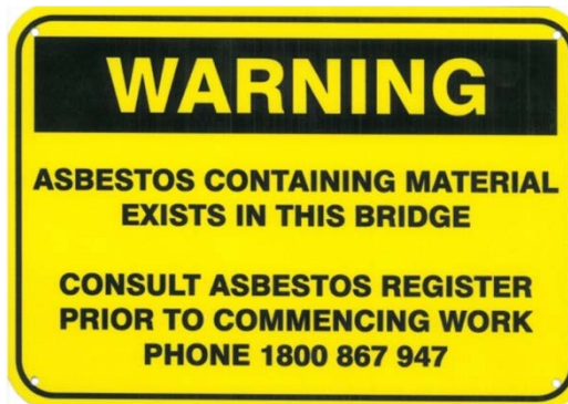
Figure 4.3.6b – Asbestos hazard warning sign
