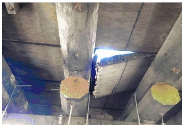
Figure 3.3.3.2b – Failure of plywood deck panel
