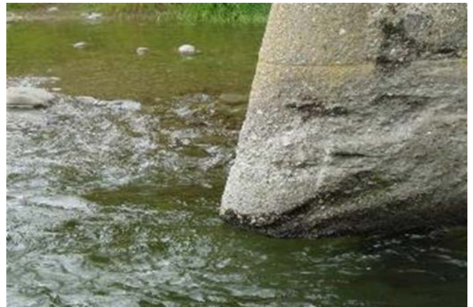
Figure 2.2.6f – Abrasion of concrete
