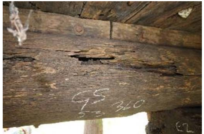
Figure 2.4.1b – Decay pocket in girder
