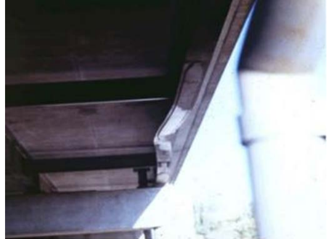
Figure 2.3.3b – Impact damage to steel beam
