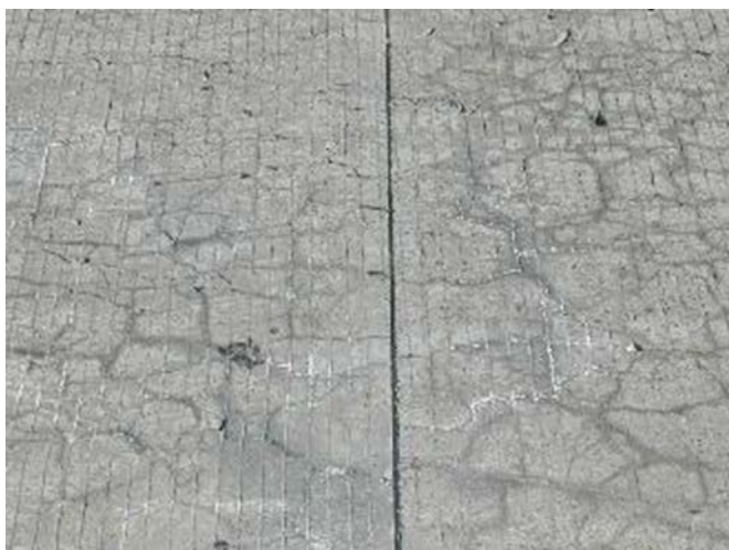
Figure 2.2.3.1b – Plastic shrinkage cracking in bridge deck
