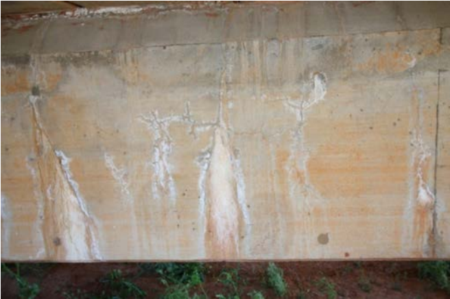
Figure 2.2.6c – Efflorescence evident on concrete headstock
