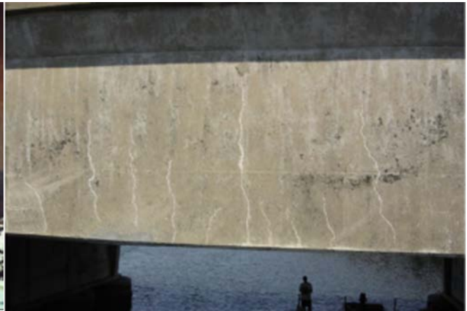
Figure 2.2.3.2b – Typical flexural cracks at mid-span of girder
