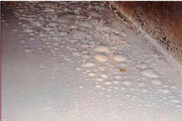
Figure 2.3.2c – Blistering of paint system
