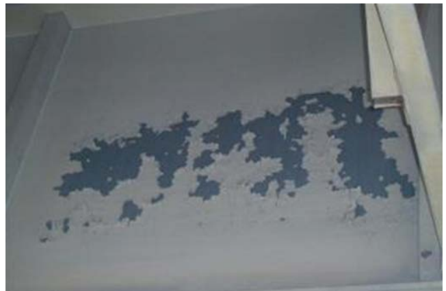
Figure 2.3.2d – Flaking of paint system
