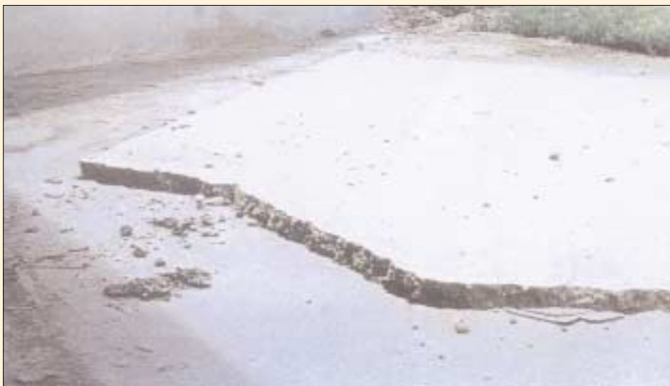
Typical apron slab crack near the wing wall slab. Note the vertical displacement across the break, and the rise of the apron slab relative to the wing wall slab.
