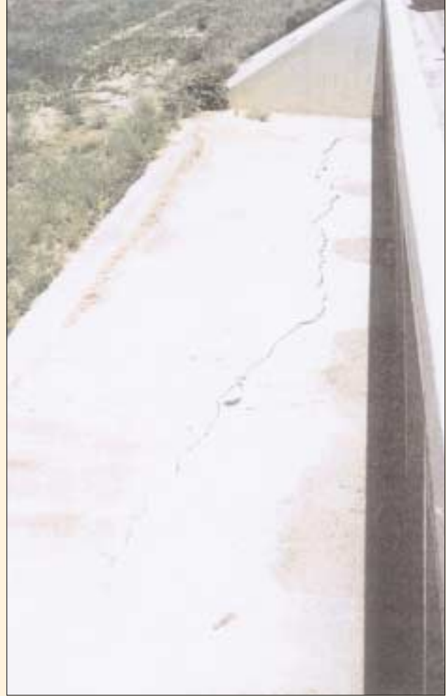
Typical crack in apron slab; note the crack stops at the slab which forms the footing of the wing wall, the apron slab has risen relative to the wingwall slab. The outer edge of the apron slab has appeared to drop and now slopes away from the culvert.
