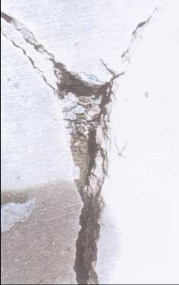
Close-up of typical crack in apron slab.
