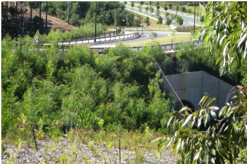
Figure C6-22: The use of vegetation around drainage structure to improve aesthetics and improve integration
