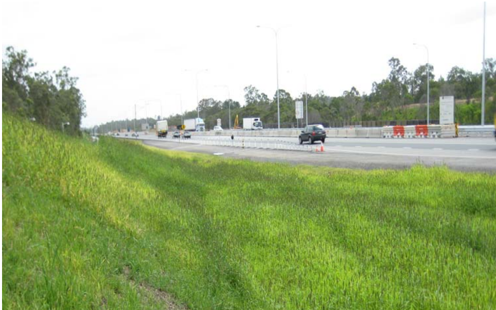
Figure C6-8: Grass seeding used as a temporary erosion and sedimentation control measure during construction
