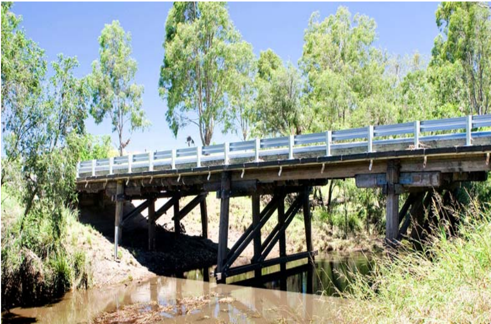
Figure C6-19: A sympathetic road crossing over a local waterway, using lightweight construction materials
