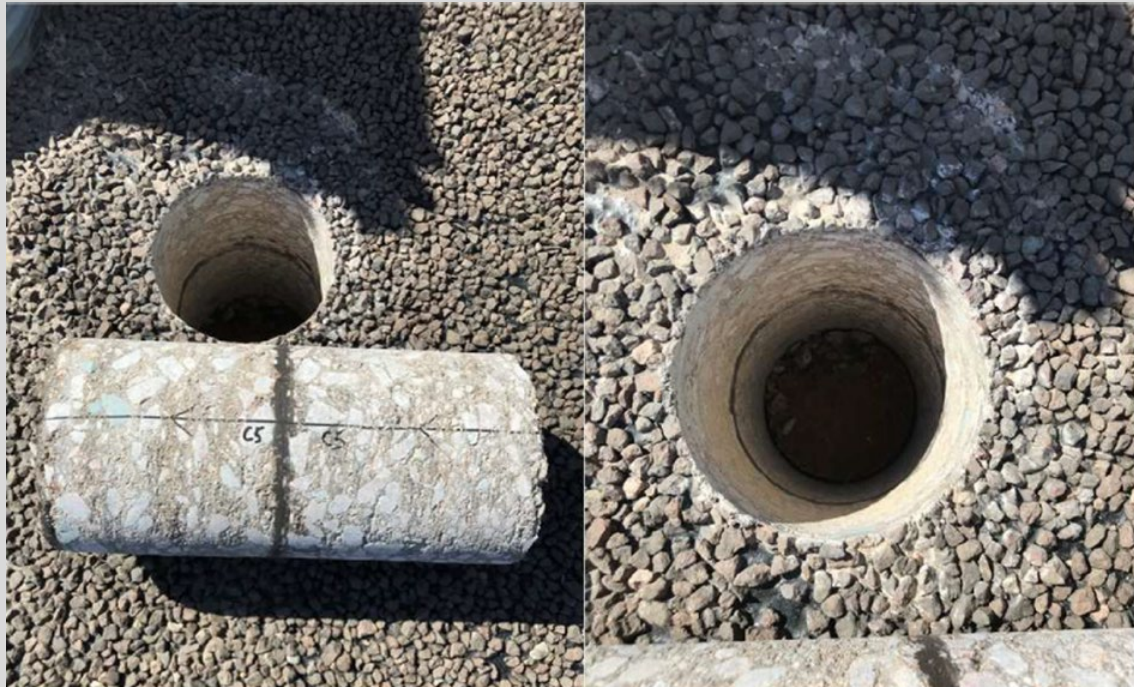
Figure 8.8.9.4.3 – Core showing the C170 spray seal interlayer bonding PMFB stabilised layers together
