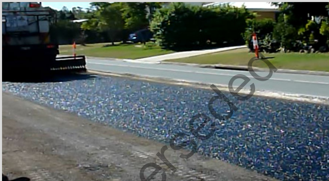
Figure 9.5.3 – Example of C170 bitumen bond coat sprayed on a prepared pavement surface
