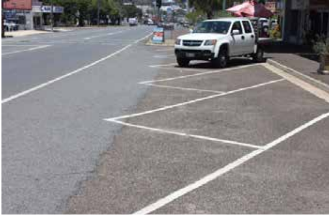
Local Government is responsible for the carriageway outside the shoulder or cycle lane where the angled parking is provided.
