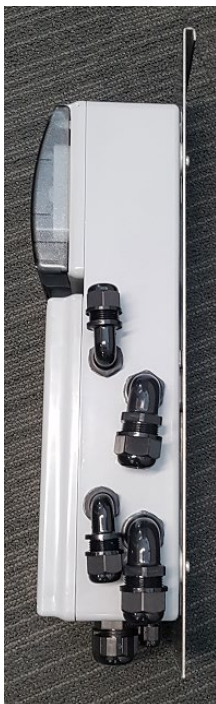
Figure 7.1(b) – Switchboard for camera side view with the backing plate and connections
