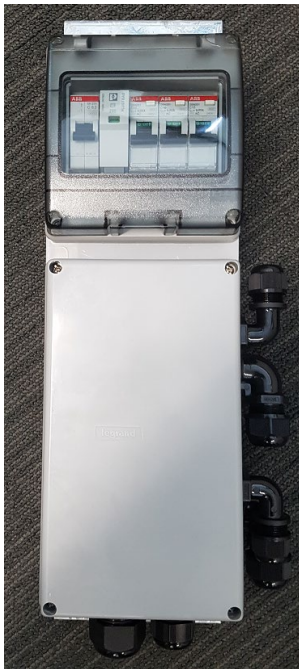
Figure 7.1(a) – Switchboard for camera front view
