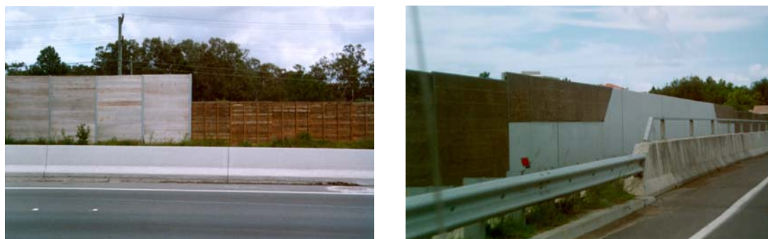
Figure 7.8.1.2 (b) - Transition between materials causing disharmony
