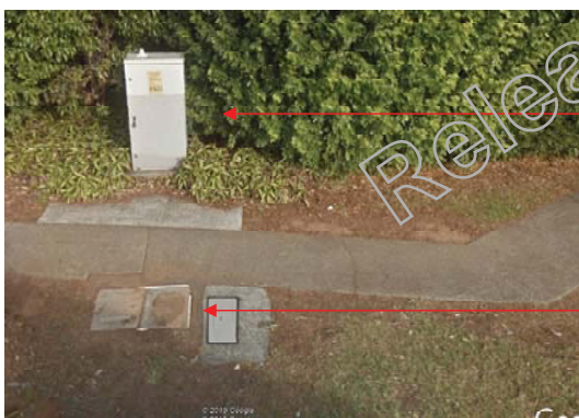
M1626 Traffic Signal Controller Existing Fibre Pit
