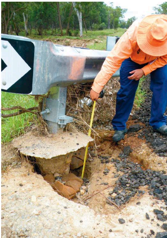
Blyth Creek – scouring around guardrail
