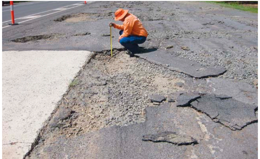
Damage caused to bitumen during the early 2010 flood
