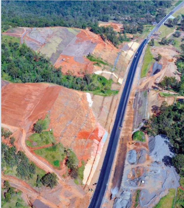
Aerial view of roadwork cuttings – South West Transport Corridor at Redbank Plains
