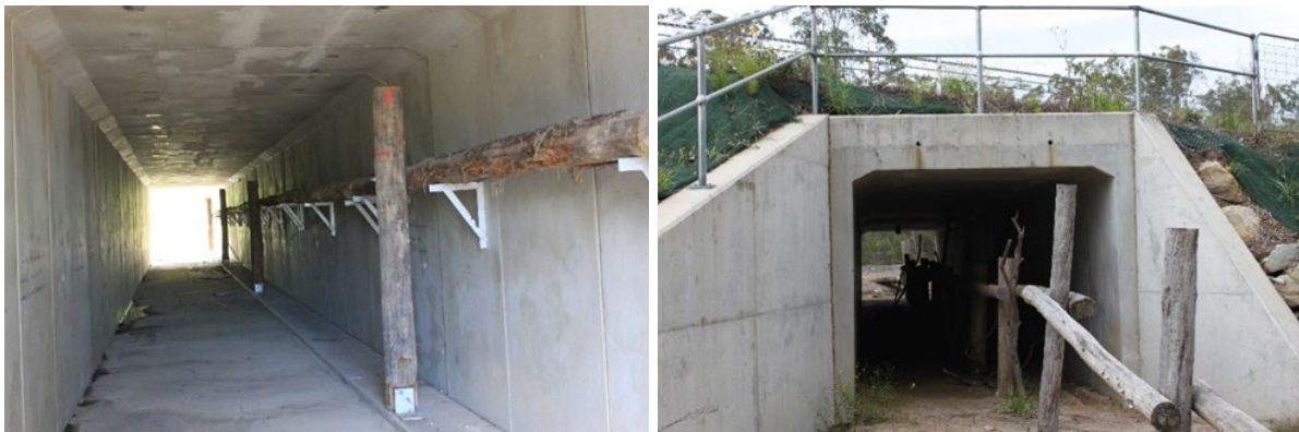
Figure 6.4(b) – Log rails in culverts under the Pacific Highway, Woolgoolga to Ballina
