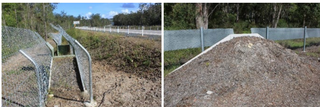
Figure 6.2.2.3 – Jump-outs for koalas on the Pacific Highway with ramps
