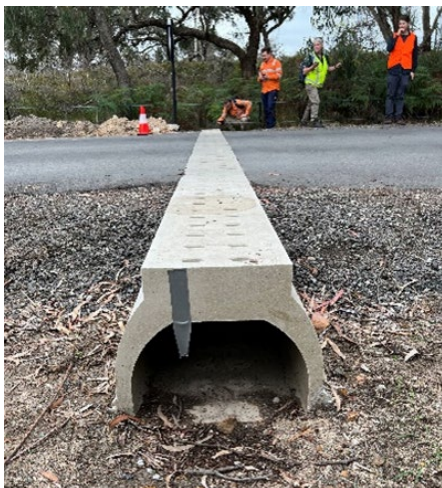
Figure 6.1.2(a) – Slotted culvert installed in Royal Botanic Gardens Cranbourne, Victoria for small mammals, reptiles, and amphibians.
