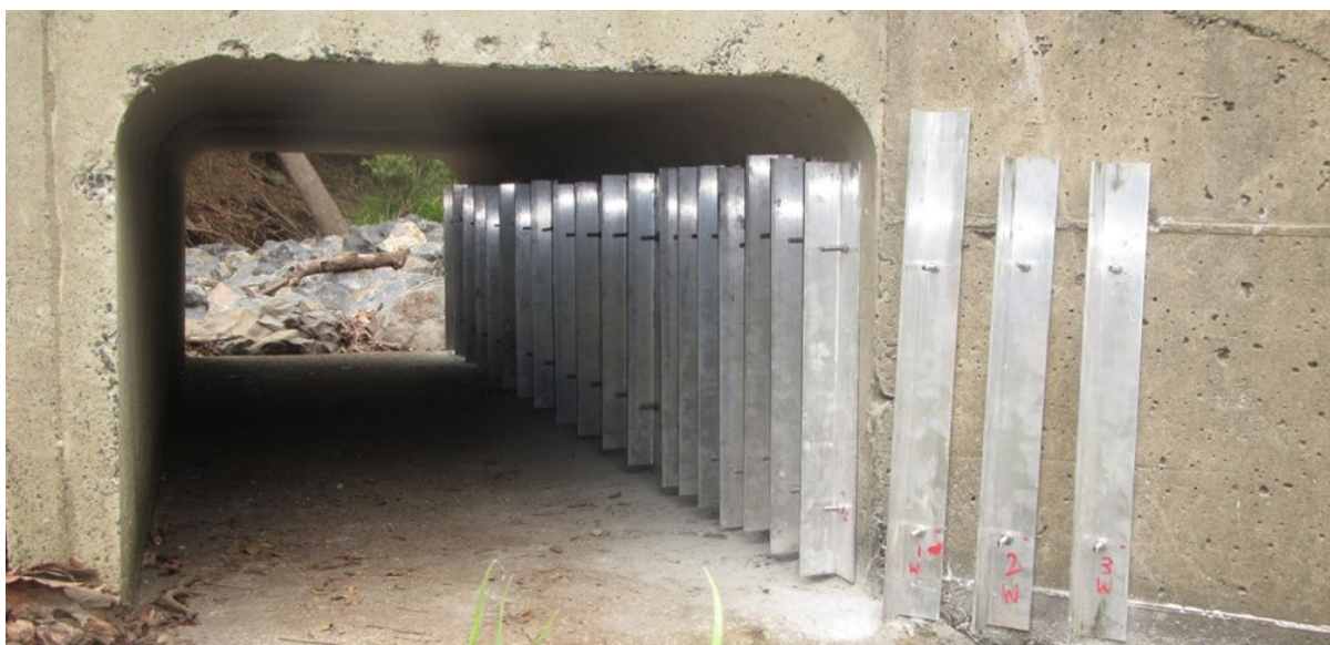
Figure 6.2 – Example of aluminium right-angle baffles installed on bankside culvert viewed from upstream
