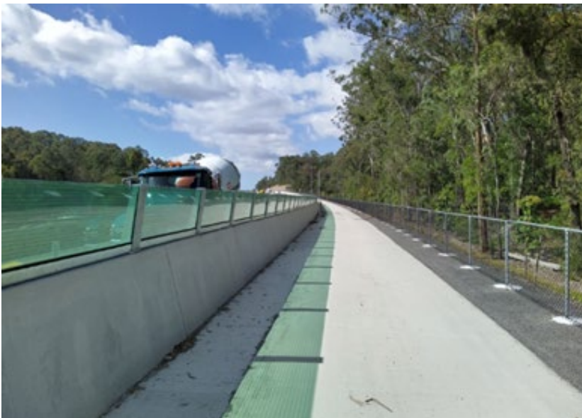
Figure 7(e) – Acrylic panels on concrete barrier designed to be a fauna exclusion barrier.
