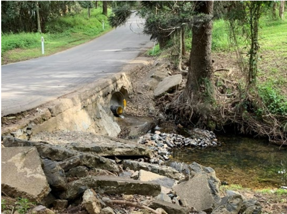
Figure 4.2(b) – Pipe culvert with perched exit under Savages Rd, Brookfield, Queensland
