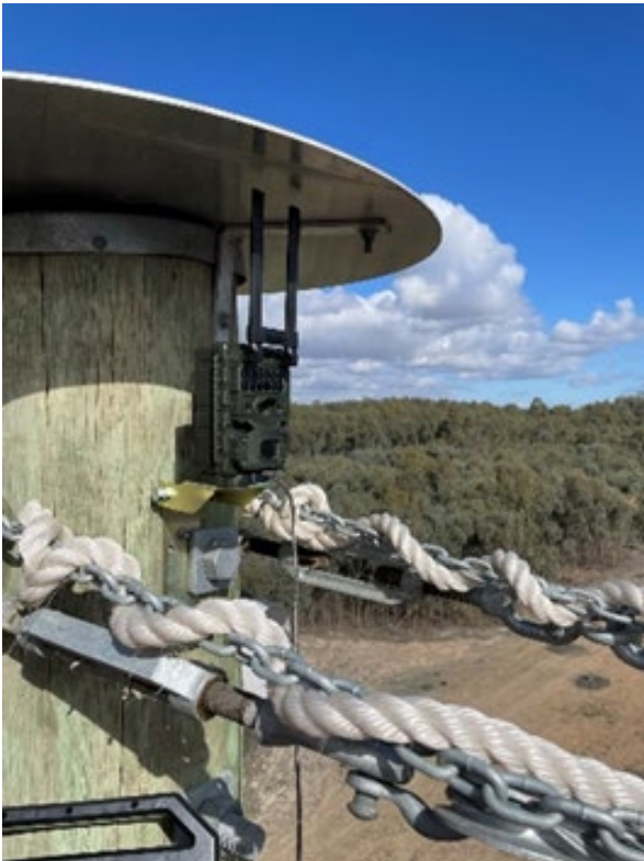
Figure 7(g) – Close-up of camera on canopy bridge below predator shield
