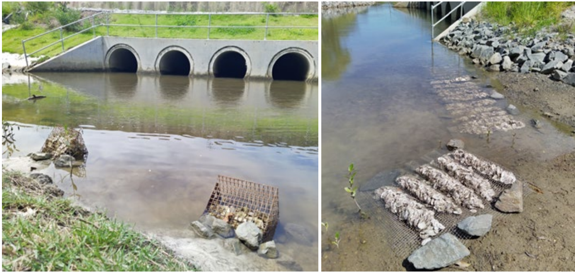
Figure 6.11(b) – Installed robust oyster baskets and quilted oyster doonas to enhance marine biodiversity
