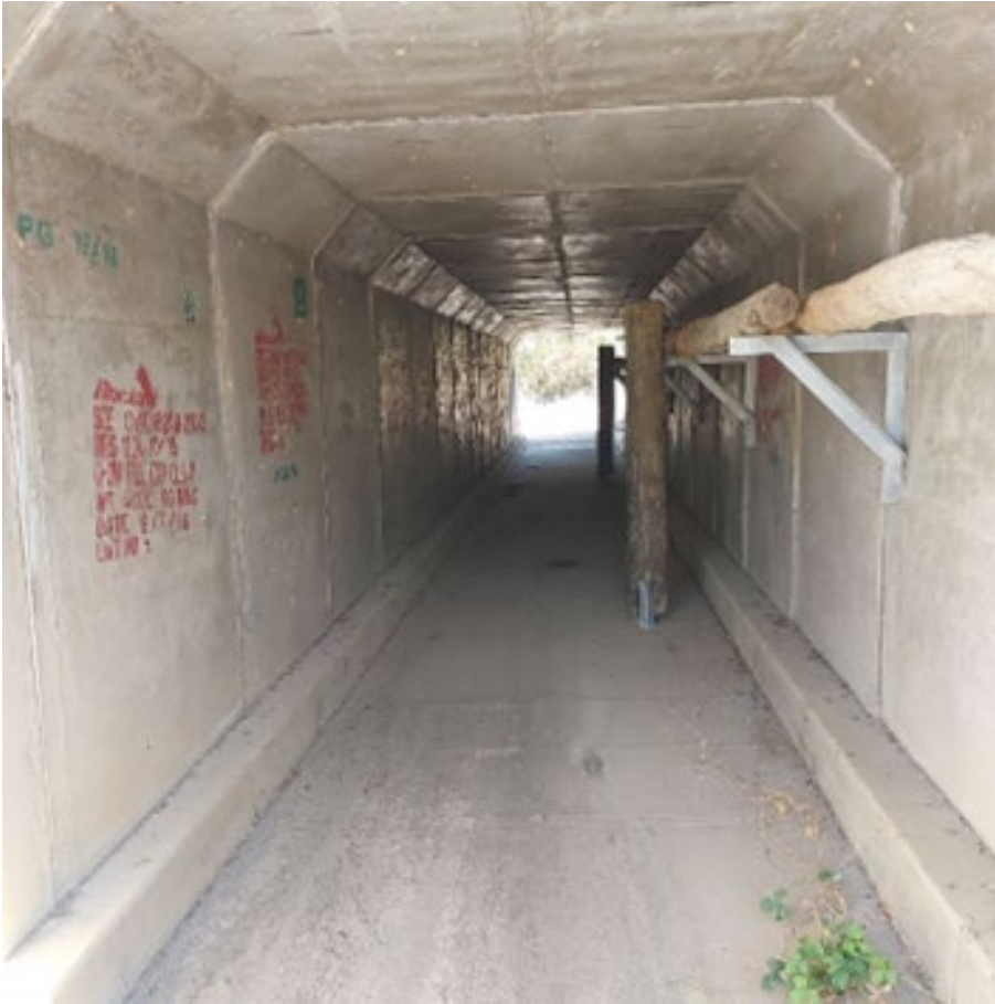
Figure 16.8(b) – Terrestrial fauna culvert with refuge poles and log rail, Eton Range (Peak Downs Highway), Queensland
