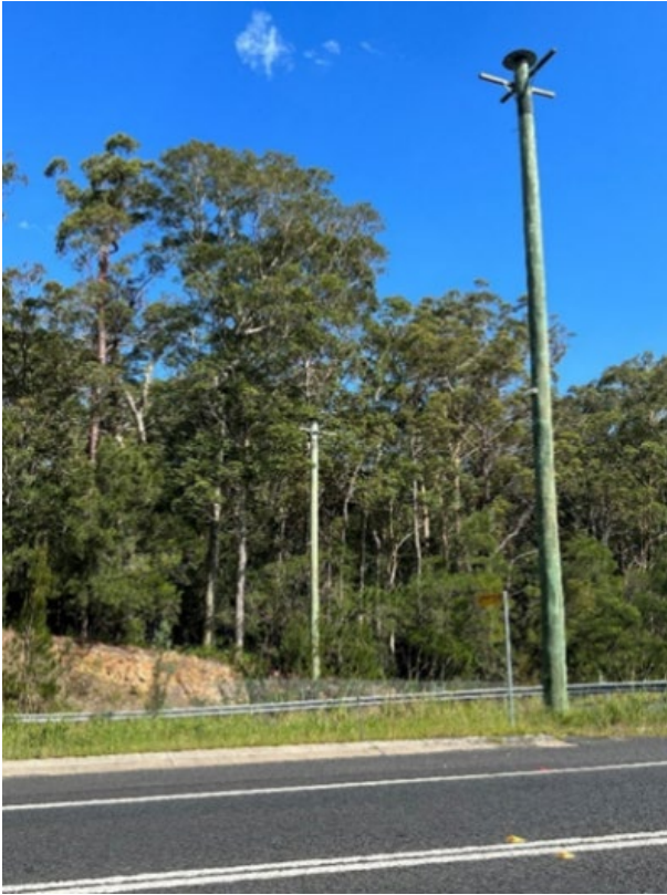
Figure 9(a) – Glider Pole in centre median and verge of Princes Highway, south coast of NSW
