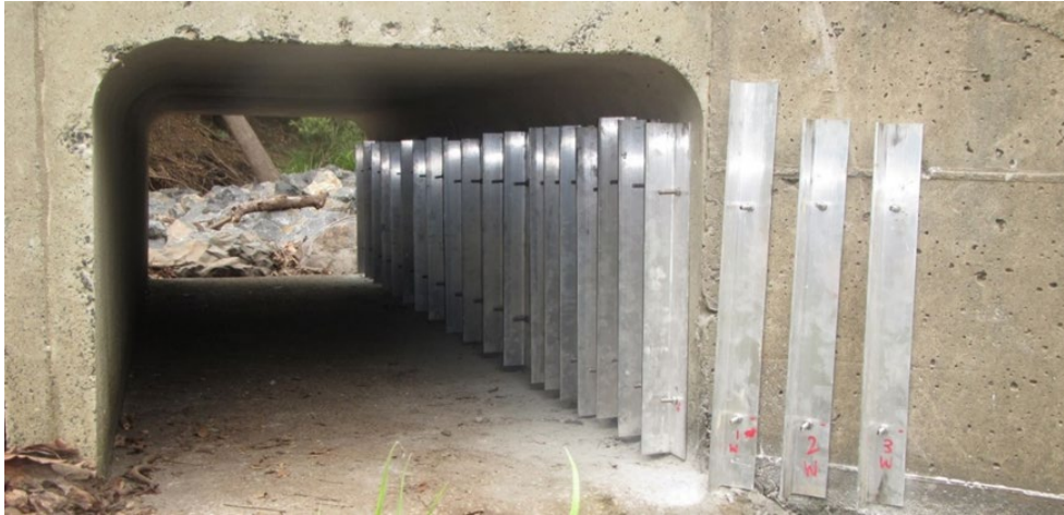
Figure 4.2(a) – Example of aluminium right-angle baffles installed on bankside culvert viewed from upstream
