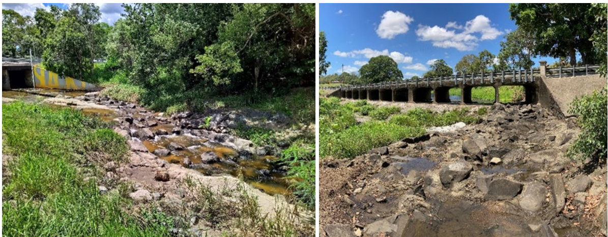
Figure 5(b) – Slacks Creek fishway (left), and Reliance Creek fishway (right)
