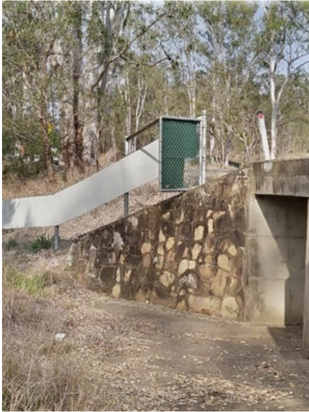
Figure 15.2(c) – Jump down on the wing-wall of a culvert on Beaudesert to Boonah Road
