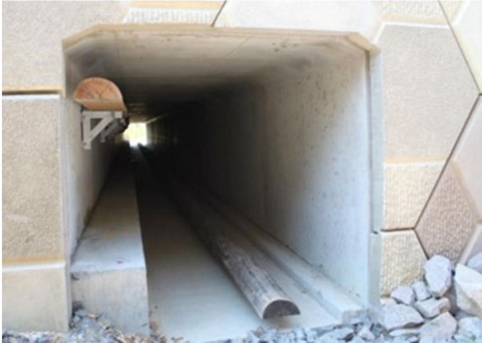
Figure 16.8(a) – Terrestrial fauna culvert under construction, with log rails at two heights and a shelf in case of flooding
