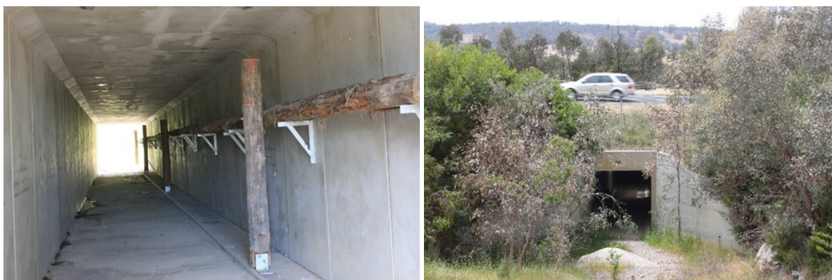
Figure 4.1 – 3.0 x 3.0 metre box culvert on Pacific Highway, Woolgoolga to Ballina (left), and 2.4 x 2.4 metre box culvert on Calder Freeway, central Victoria (right)
