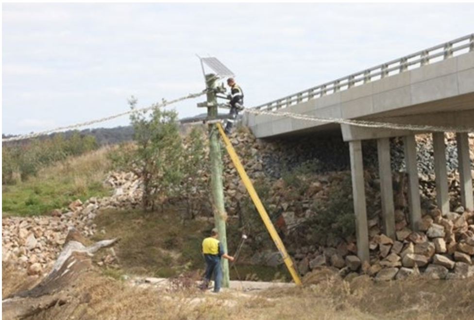
Figure 8(a) – Under-road canopy bridge during camera installation on the Hume Freeway, NSW
