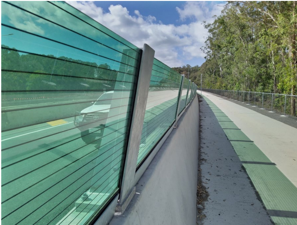
Figure 14 – Safety barrier topped with perspex barrier which functions as fauna exclusion fencing
