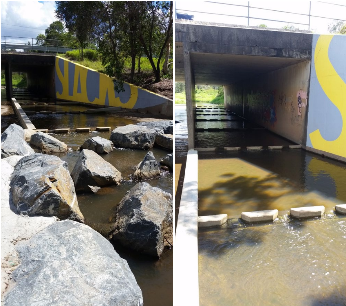
Figure 5(a) – Slacks Creek rock ladder and baffles (left), and Slacks Creek baffles (right)
