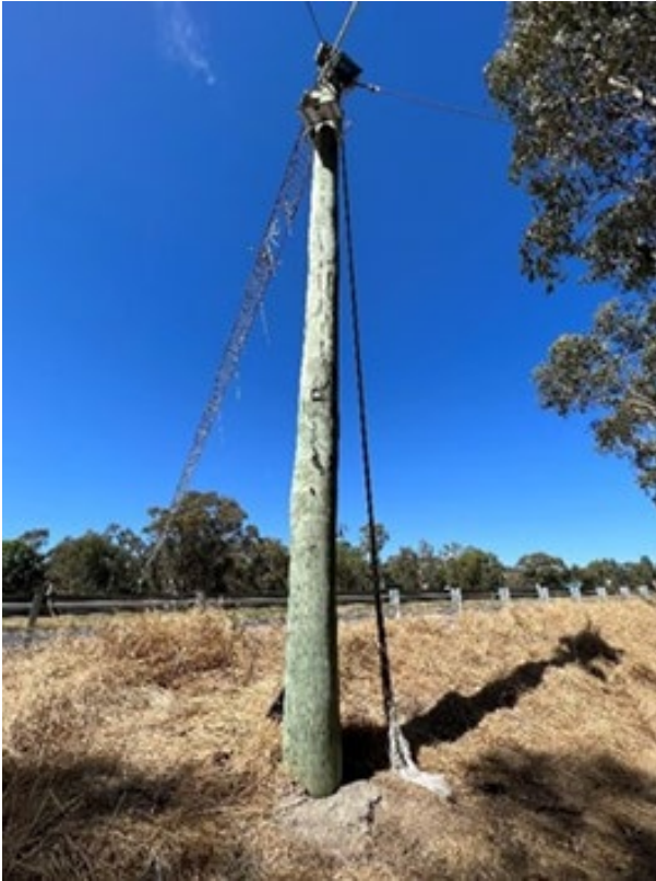
Figure 7(f) – The feeder rope of this canopy bridge has failed because the branch it was connected to has broken off
