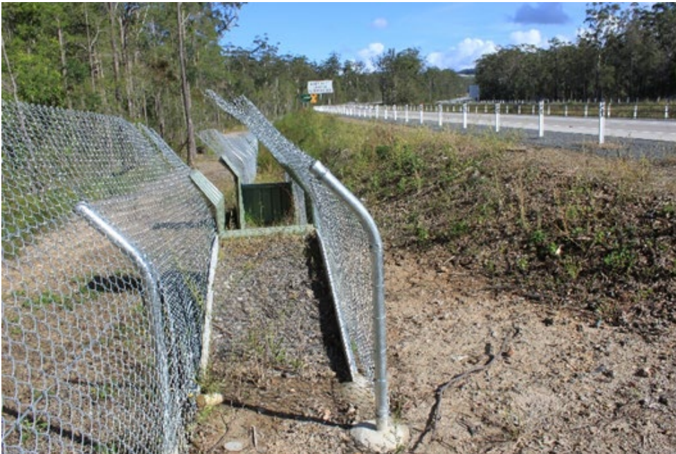
Figure 15.2(b) – Escape ramp on the Pacific Highway
