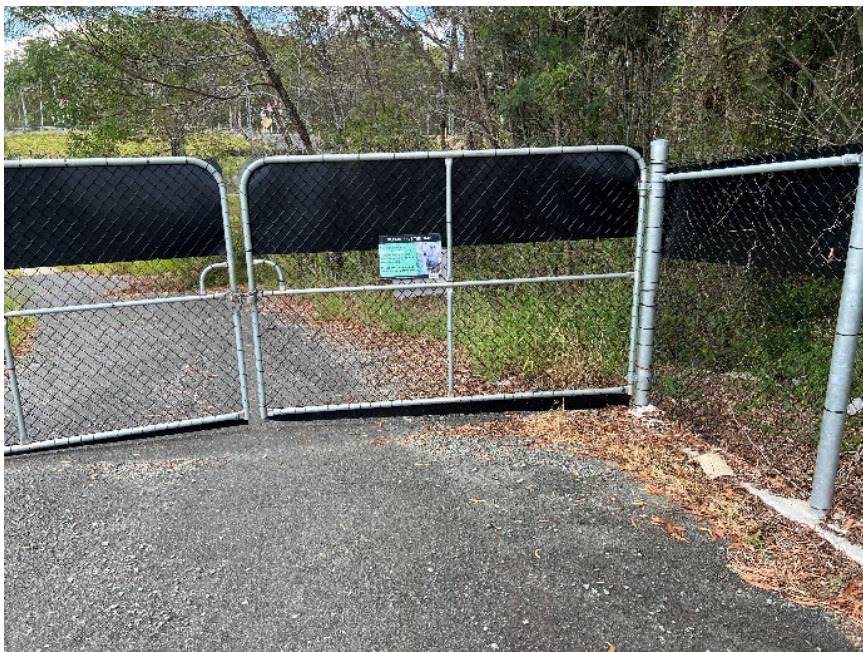
Figure 5.3.3(d) – Gaps under and between gates are weak points in fence systems and can allow animal movement.
