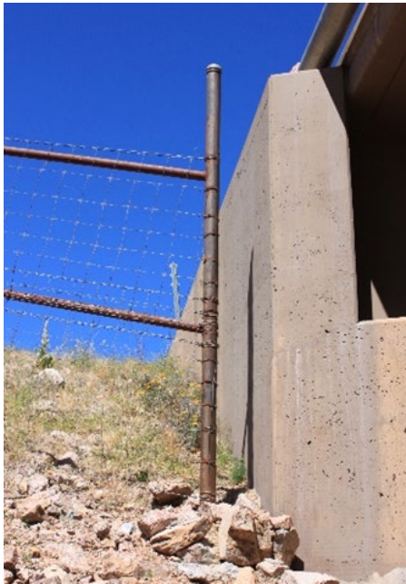
Figure 5.3.3(e) – Gap between fence and bridge abutment that animals may pass through are to be avoided
