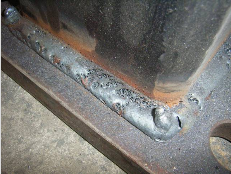
Figure 10.4.7.2(d) – Welding porosity
