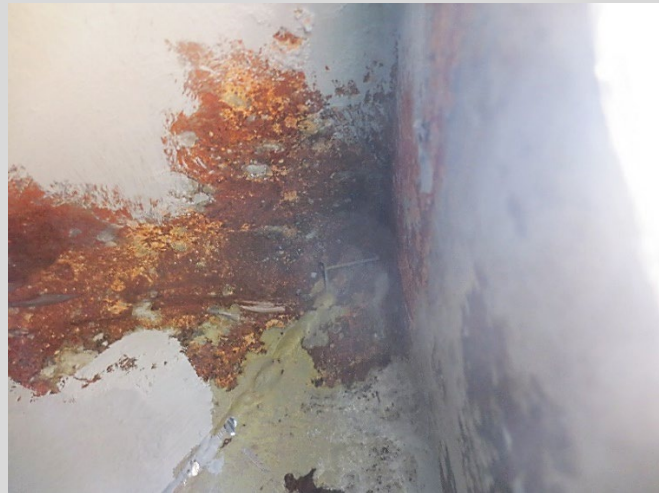
Figure 11.2.3(c) – Insufficient venting and drainage
