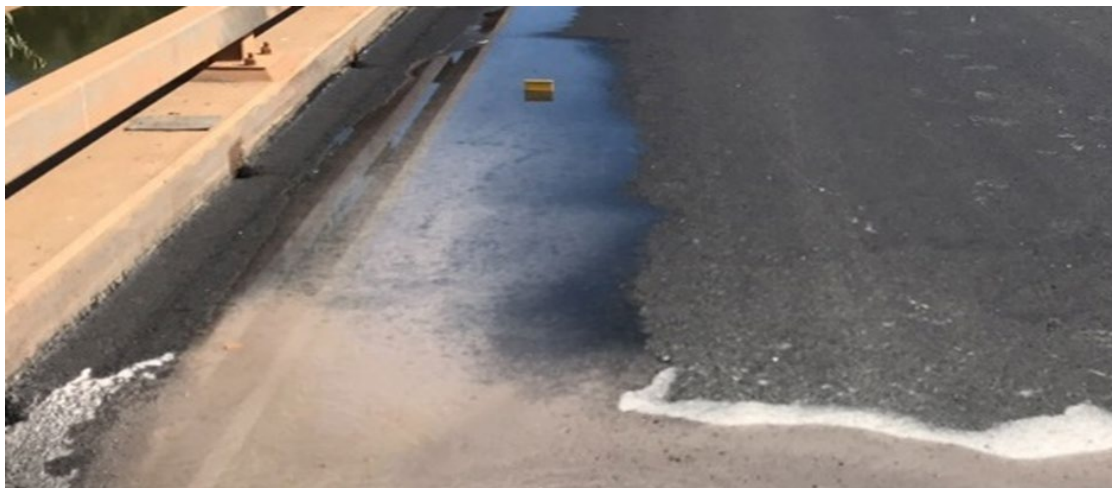
Figure 6.6(f) – Uncompacted asphalt DWS edge resulting in poor surface drainage
