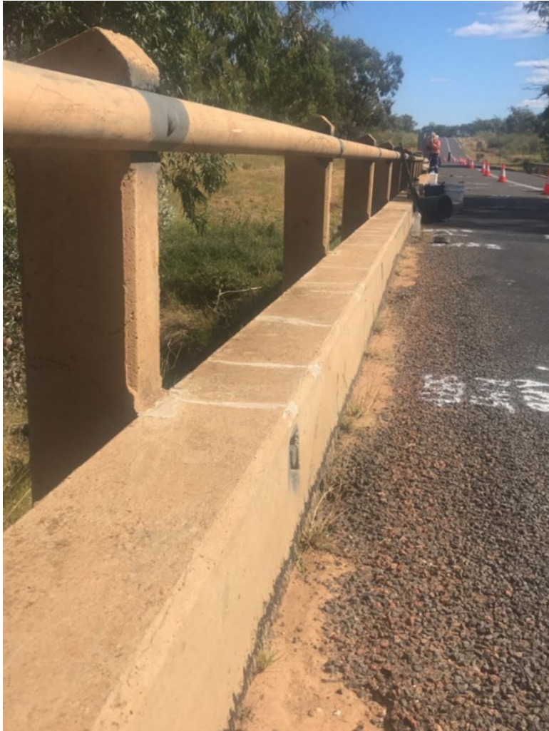
Figure 6.6(b) – Bridge railing setback from the inside face of the concrete kerb
