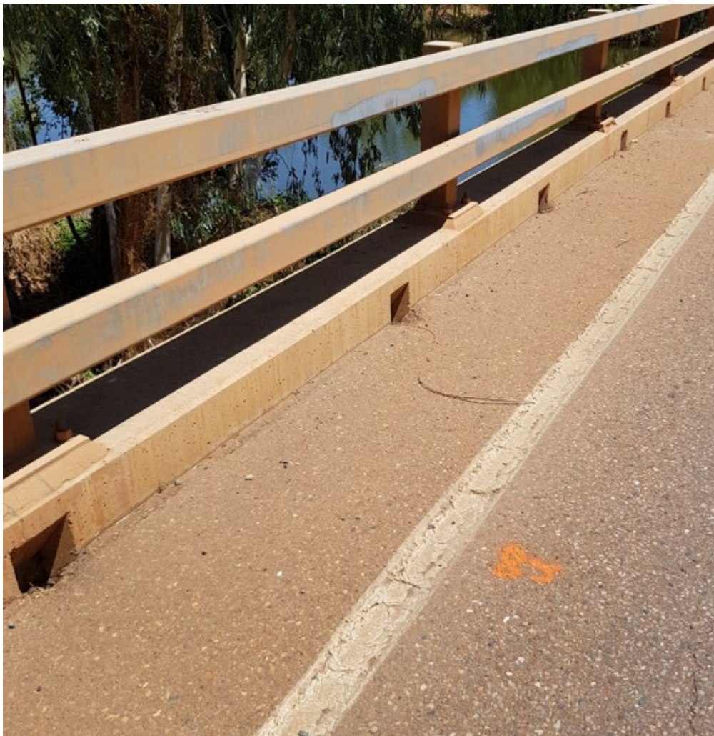
Figure 6.6(a) – Bridge railing flush or intruding beyond the inside face of the concrete kerb
