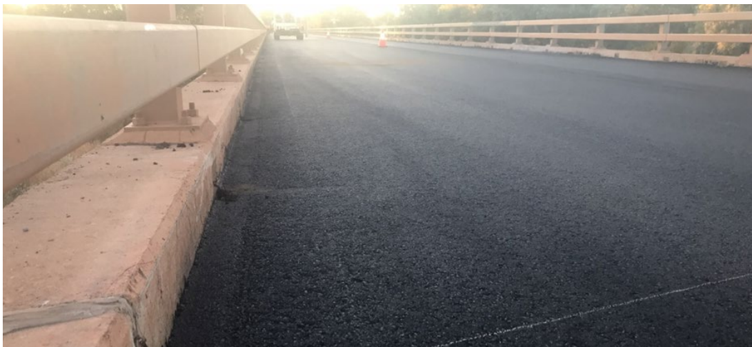
Figure 6.6(e) – Uncompacted asphalt DWS resulting in a stepped asphalt strip along the concrete kerb
