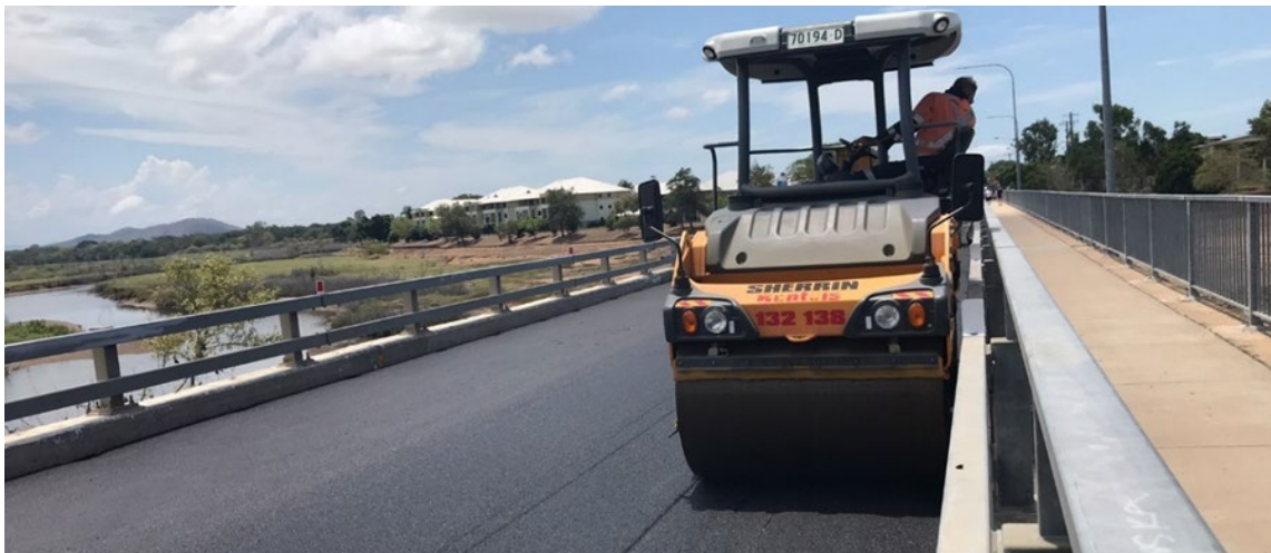
Figure 10.11(b) – Asphalt compaction along the edges – bridge railing with adequate compaction clearance
