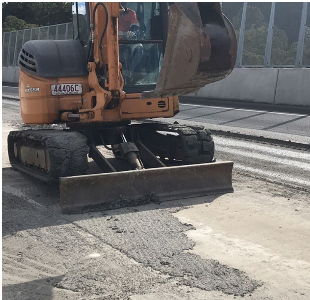
Figure 10.4(e) – A small excavator using a blade attachment to remove residual asphalt DWS
