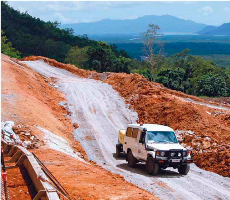
Early works on the Bruce Highway realignment north of the Cardwell Range
