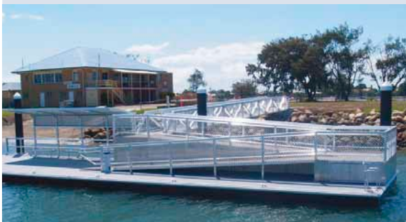
The new custom-built pontoon at Manly Boat Harbour will benefit people with disabilities
