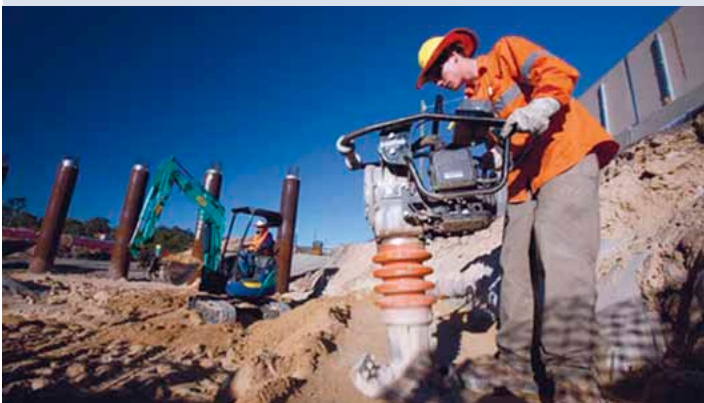
One of our 'Constructive Kids' trainees at work on the Ipswich Motorway upgrade
