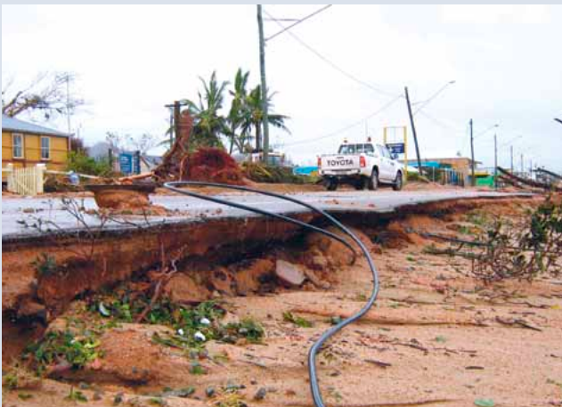
Emergency response crews inspect damage to the Bruce Highway at Cardwell following Severe Tropical Cyclone Yasi
