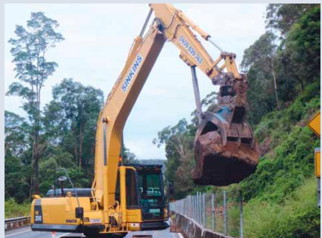
Boulders, weighing many tonnes, were dislodged by land slips at Cunningham's Gap
