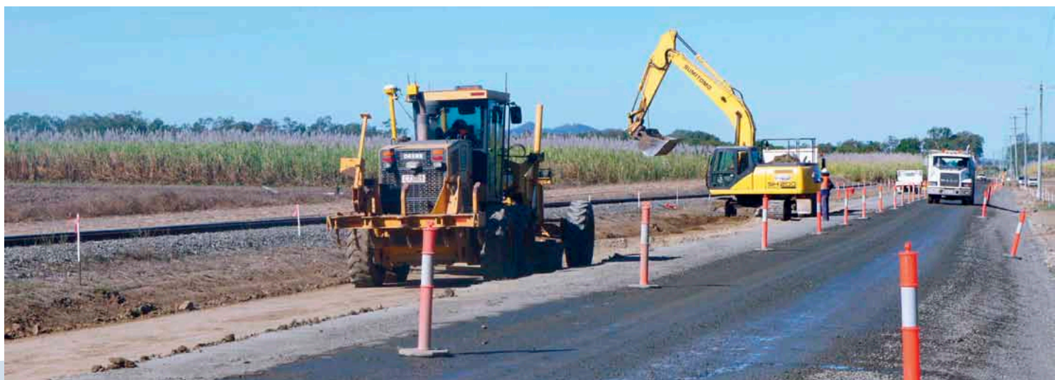
Subgrade treatment on Miran–Eton Road in the Mackay/Whitsunday region as part of the Transport Network Reconstruction Program
