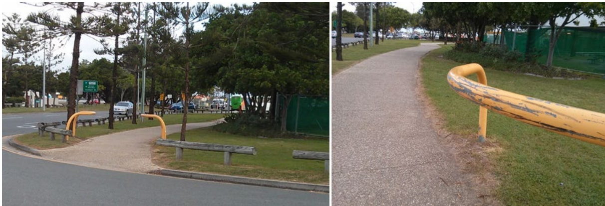
Figure C.16 – Damage which indicates evidence of insufficient passing width
