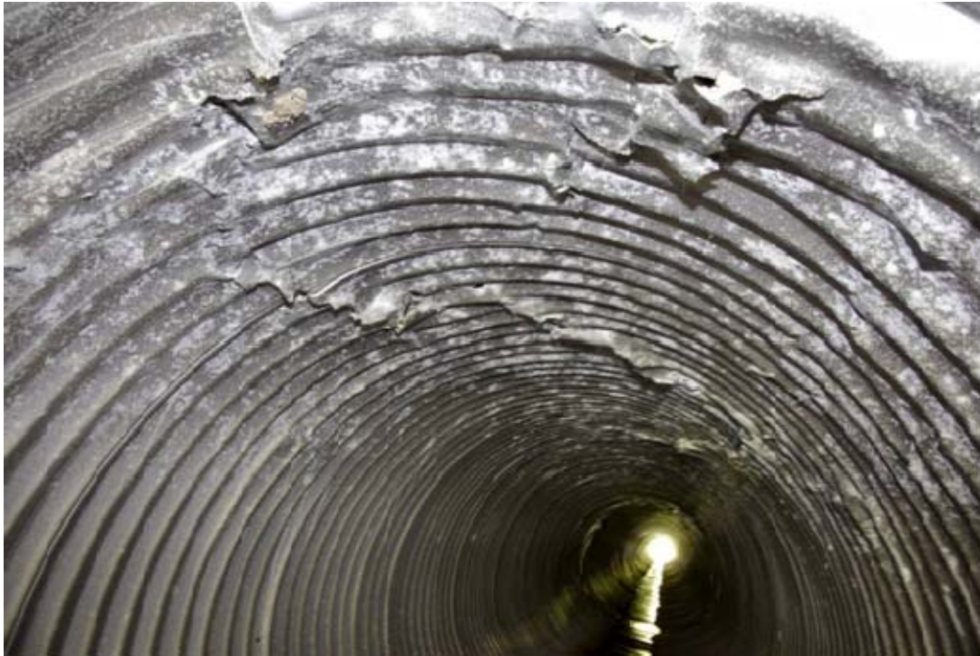
Figure 9 - An aluminium culvert exhibiting local crushing due to corrosion of the upper portion of the culvert
